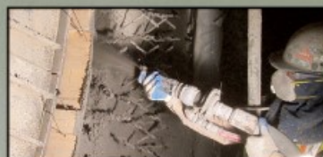
BOTTOM: Using two different activators, walls and roofs were lined without an issue.
