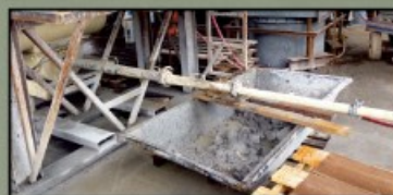
TOP: Even with pipe reductions & 150 ft vertical hose heights, the pumping and shooting was done without one problem!
