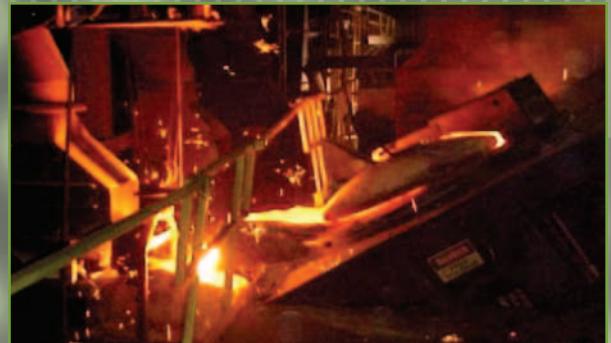
Reliable, consistent and cost effective refractory performance in the coreless furnace requires a "systems approach" that involves the refractory components and installation process.
