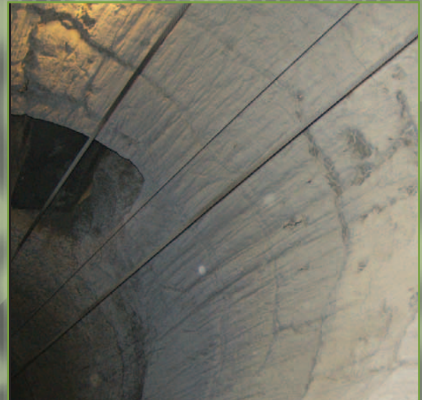
Prior to the veneering process, the original lining should be free of most debris and worn refractory. This is an example of an excellent clean up prior to gunning.
