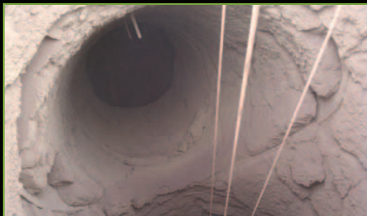
BEFORE gunning UNI-BRADE AR-85 on the joint where the crossover meets the upperstack.
