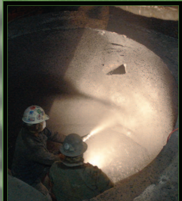
To extend the furnace campaign and eliminate an annual brick reline, UNI-SHOT 400 is shotcreted into a vertical channel iron holder in the Northeast.
