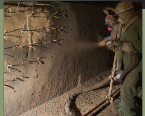
UNI-GUN RF-FS RG product installed in ash hopper.
