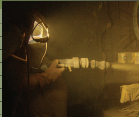
UNI-GUN RF-70 RG installed in taconite plant.
